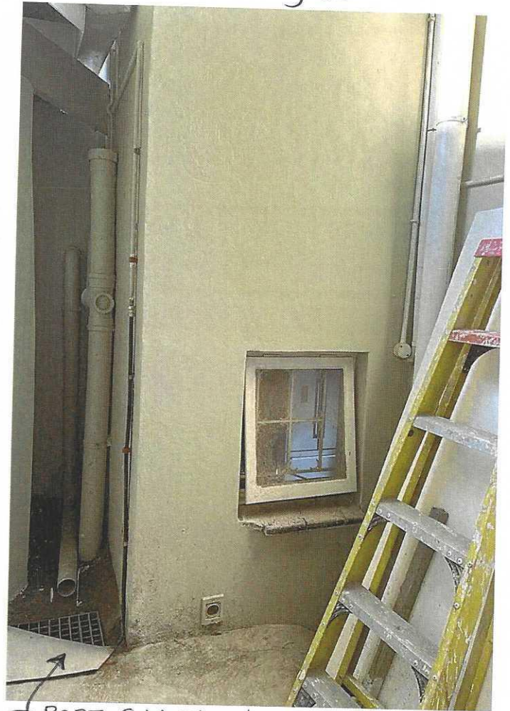
PART S.W. Elevation - DIFFICULT TO ACCESS.
