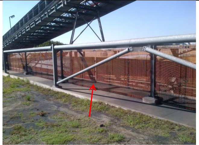
b) Conveyor Belt turnover point near the Syferfontein Bunker
