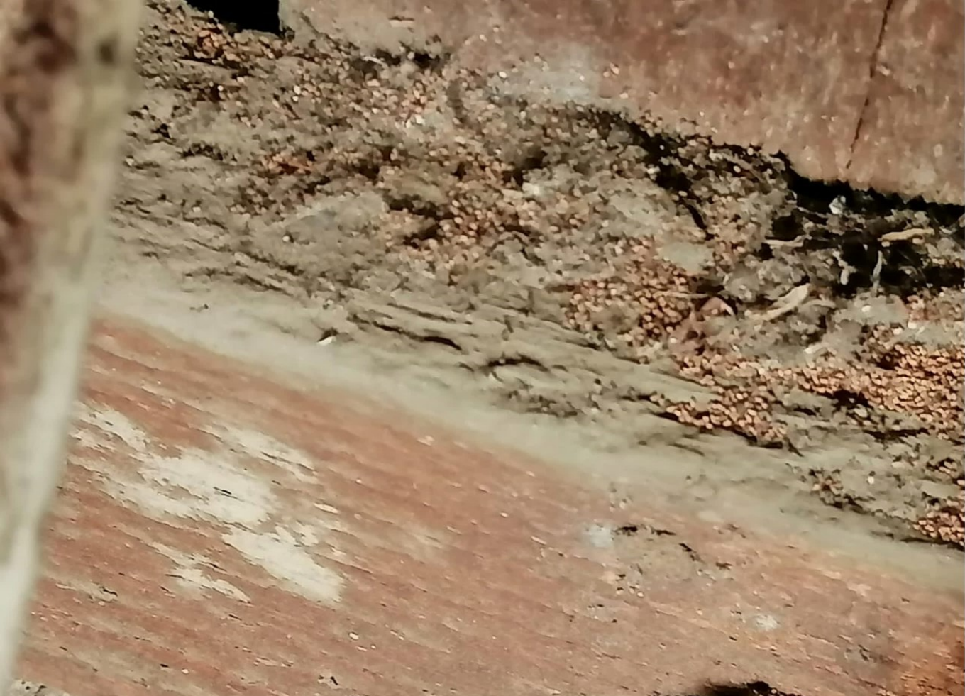
Damaged timber trusses.
