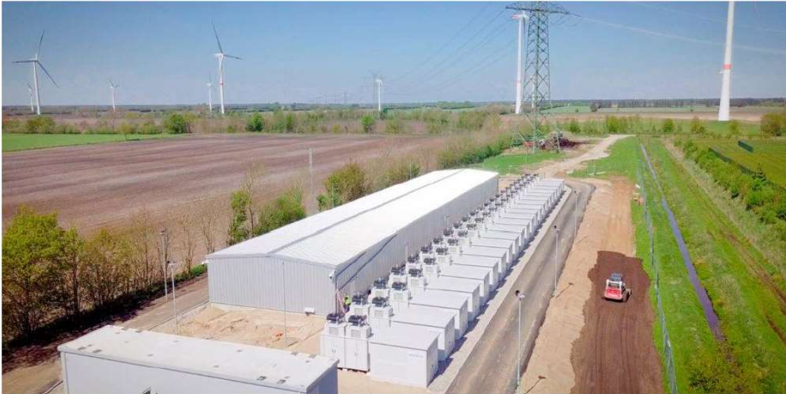
Figure 1.2: Typical Containerised Battery Energy Storage Facility
