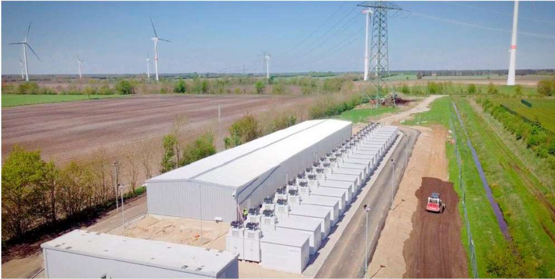
Figure 1.2: Typical Containerised Battery Energy Storage Facility
