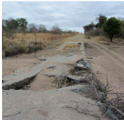
Damaged road surface.
