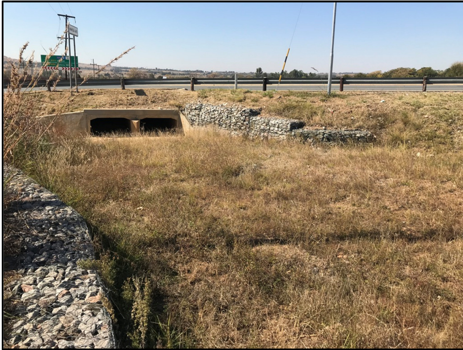
Photo 5: Stormwater drain system in northeast corner of site (Mimosa St & 1st Ave intersection)
