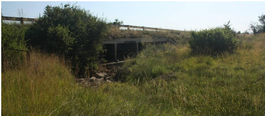
Figure 6: View of the seasonal stream 3 in the northern portion of the pipeline route. The stream will be crossed by the pipeline and is in a good condition, utmost care must be taken to keep the impact on the stream to a minimum.
