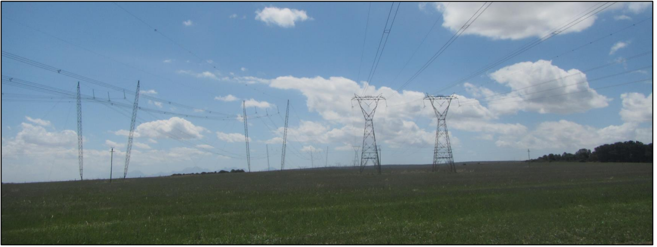
View towards the northwest in the middle of the power line route.
