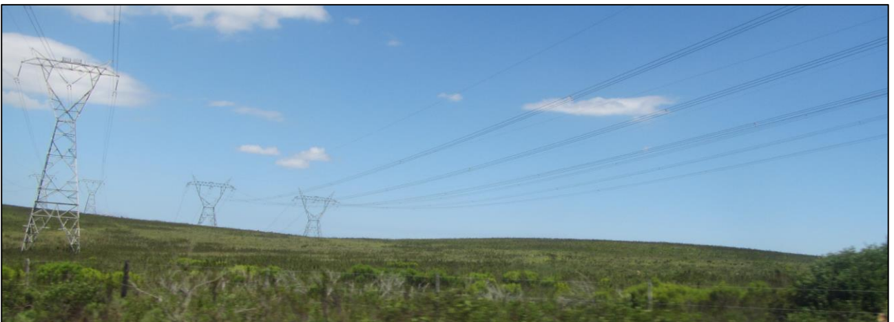
View towards the southeast along the powerline route to the substation at its north-western end as seen from the R327.
