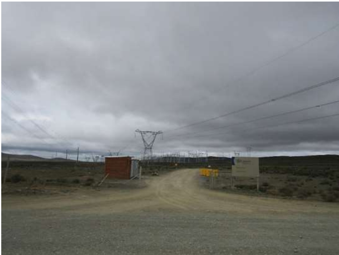
Figure 3-8: Komsberg substation (source: SiVEST, 2021)
