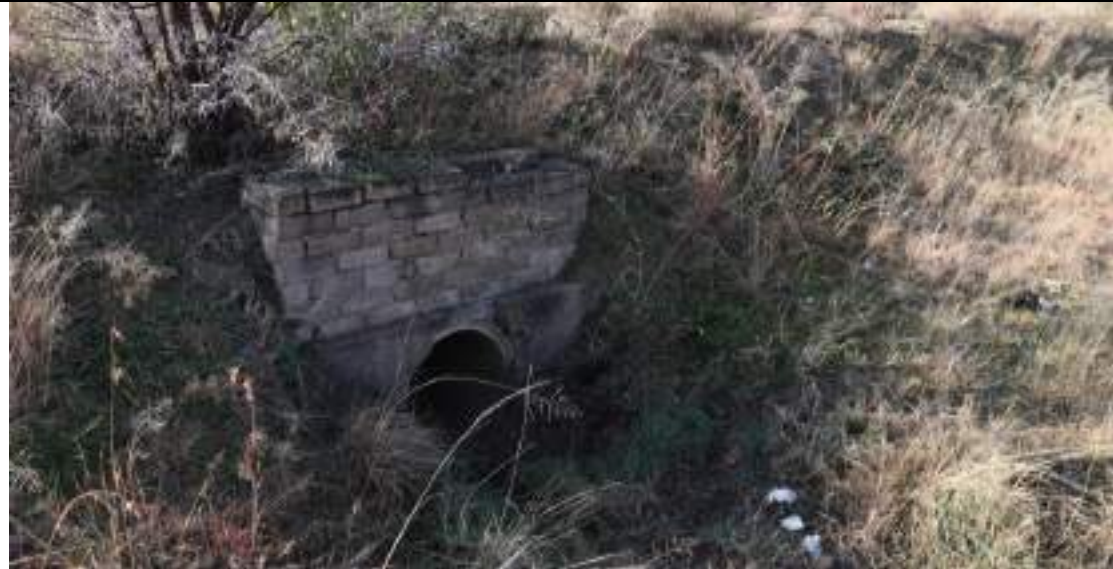
View of the culver crossing of the stream. This will clearly affect the natural flow and flooding regime of the stream.
