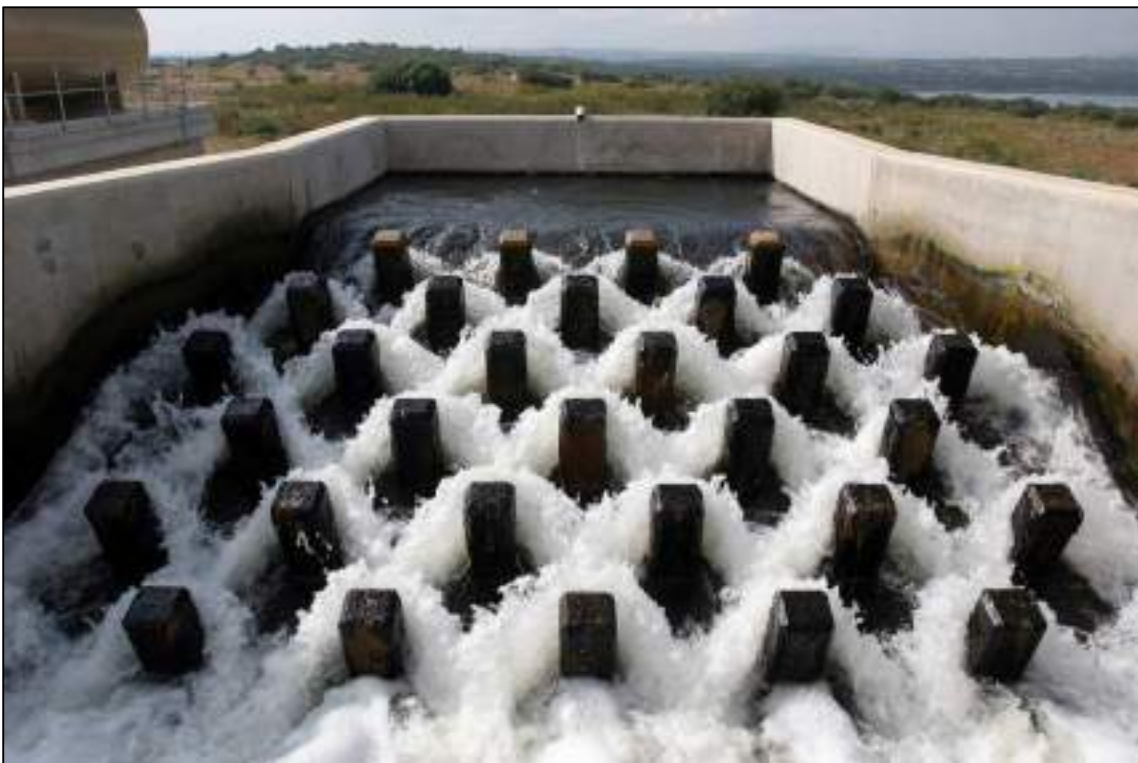
Example of the working of an energy breaker system at a pump outlet.
