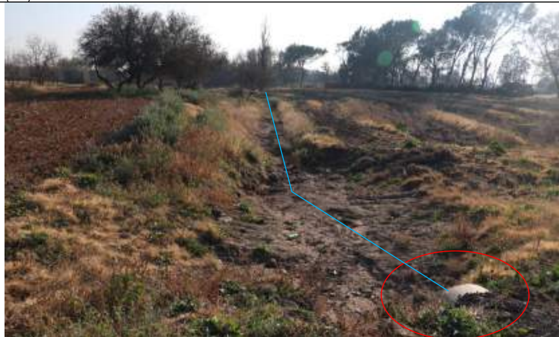
View of the culvert at the crossing (red) with the canalised section of the stream inbetween orchards and crop fields.
