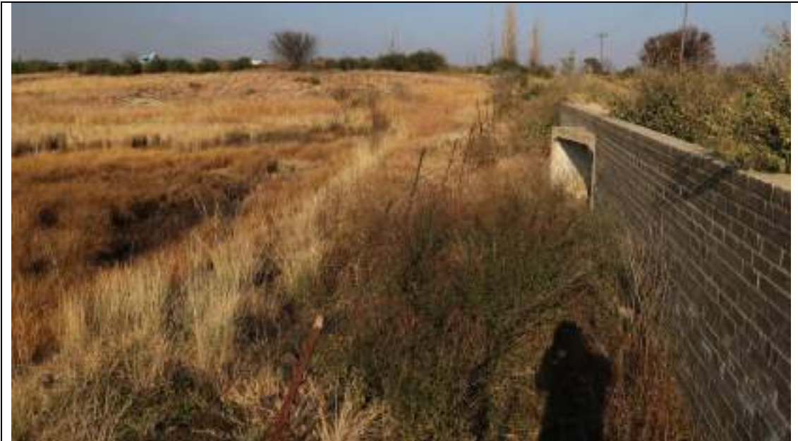
View of the culvert over the stream at the point of crossing. This also contributes to modification of the flow and flooding regime and ponding upstream of the culvert.
