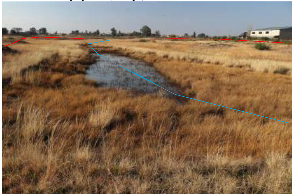
View of the stream upstream of the point of crossing. Note clear ponding caused by the road crossing. The flood bench is also quite visible here (red).
