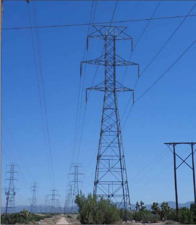
Figure 5-9: 132kV/275kV powerline double circuit suspension towers
