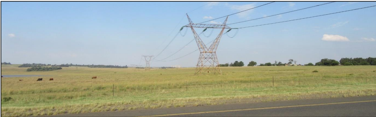
Figure 6-42: 400 kV line traversing N11 approximately 6 km south of Ermelo
