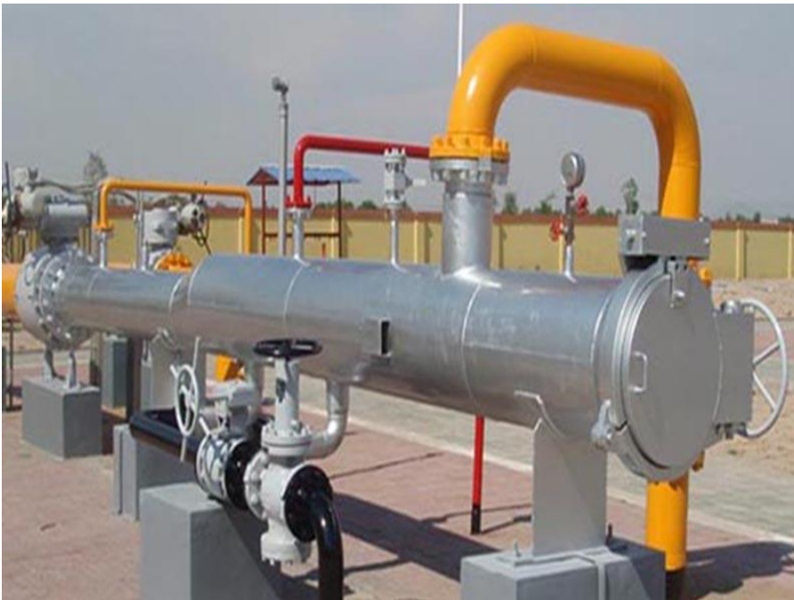
Figure 3-3 – Pig launcher/receiver for a natural gas pipeline (oilgasfacility.com)
