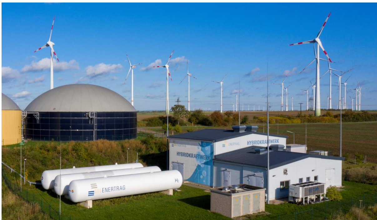
Figure 2-4: Closer View of Electrolyser Housing and Storage Tanks
