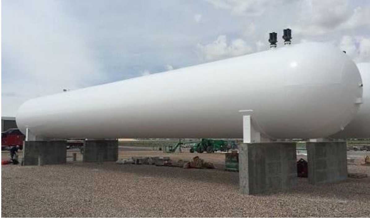
Figure 2-15: Bullet storage tank (ammonia storage)
