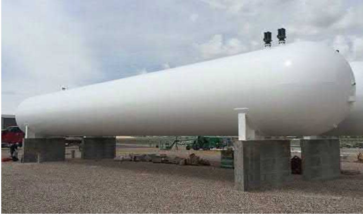
Figure 2-15: Bullet storage tank (ammonia storage)
