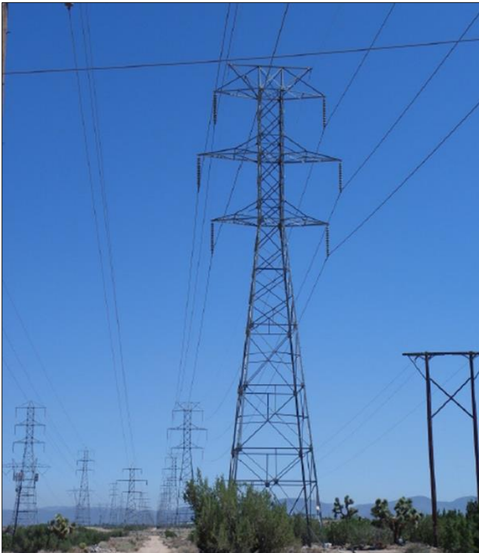
Figure 5-5: 132KV/275KV Powerline Double Circuit Suspension Towers
