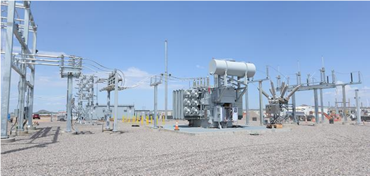
Figure 4-3: Example of substation
