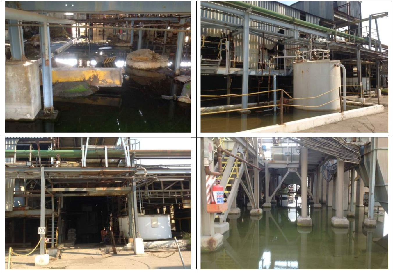
2 – Filtration Plant Area: Looking in a Easterly direction from the centre of the site being demolished.
