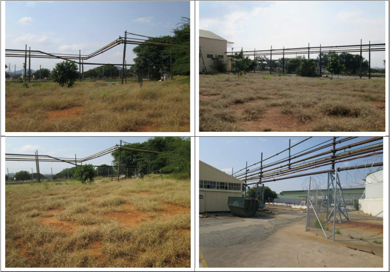
8 – Redundant Pipe Line Infrastructure: Looking in a North Westerly direction from the centre of the site being demolished
