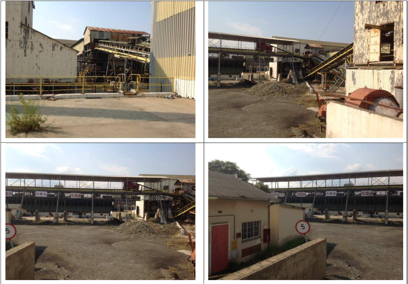
6 – Crusher Plant Area: Looking in a Southerly direction from the centre of the site being demolished.
