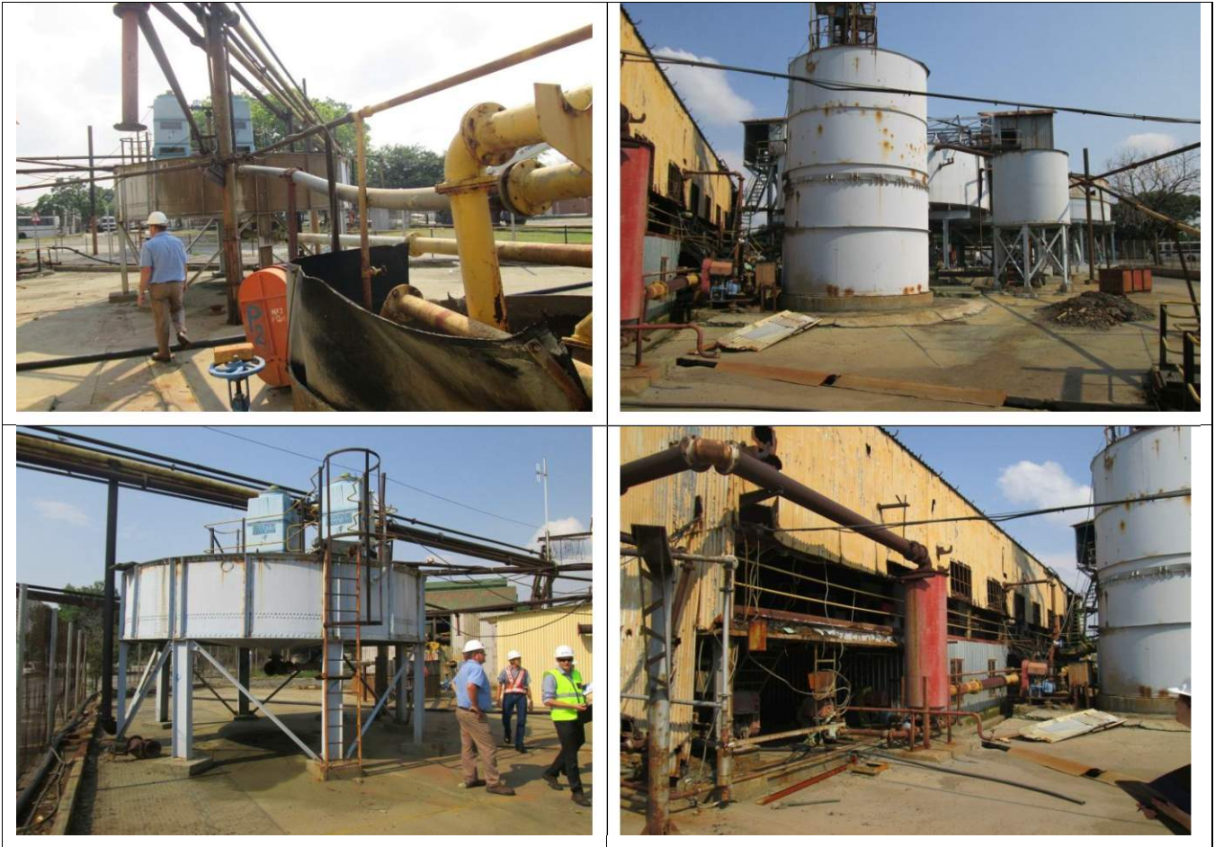
7 – Thickener Plant Area: Looking in a North Westerly direction from the centre of the site being demolished.
