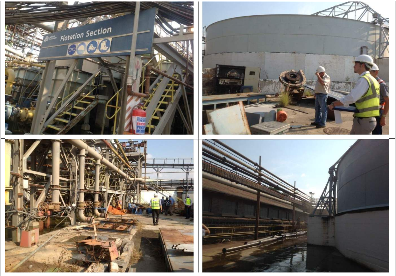
1 – Flotation Plant Area: Looking in a Westerly direction from the centre of the site being demolished.
