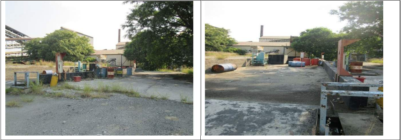
5 – Storage of Hazardous Oil: Looking in a South Easterly direction from the centre of the site being demolished.
