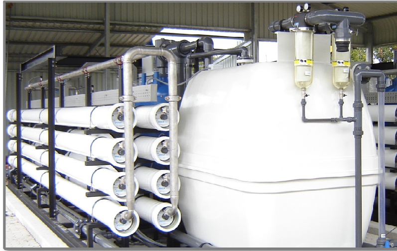
Figure 2-1: CIP Tank with RO vessels
