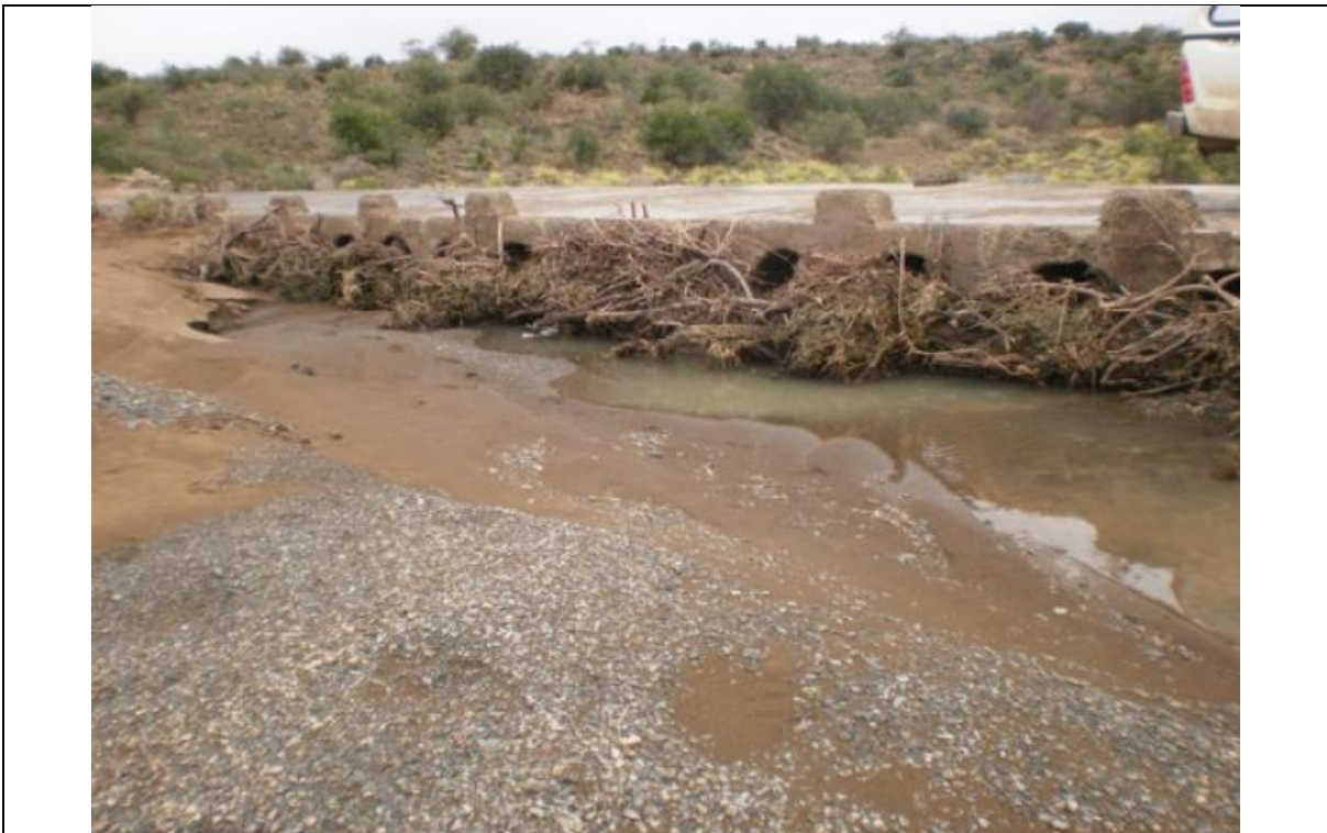
Figure 1: Crossing 7 taken from downstream. Note pipes on right hand side are dry due to blockage.
