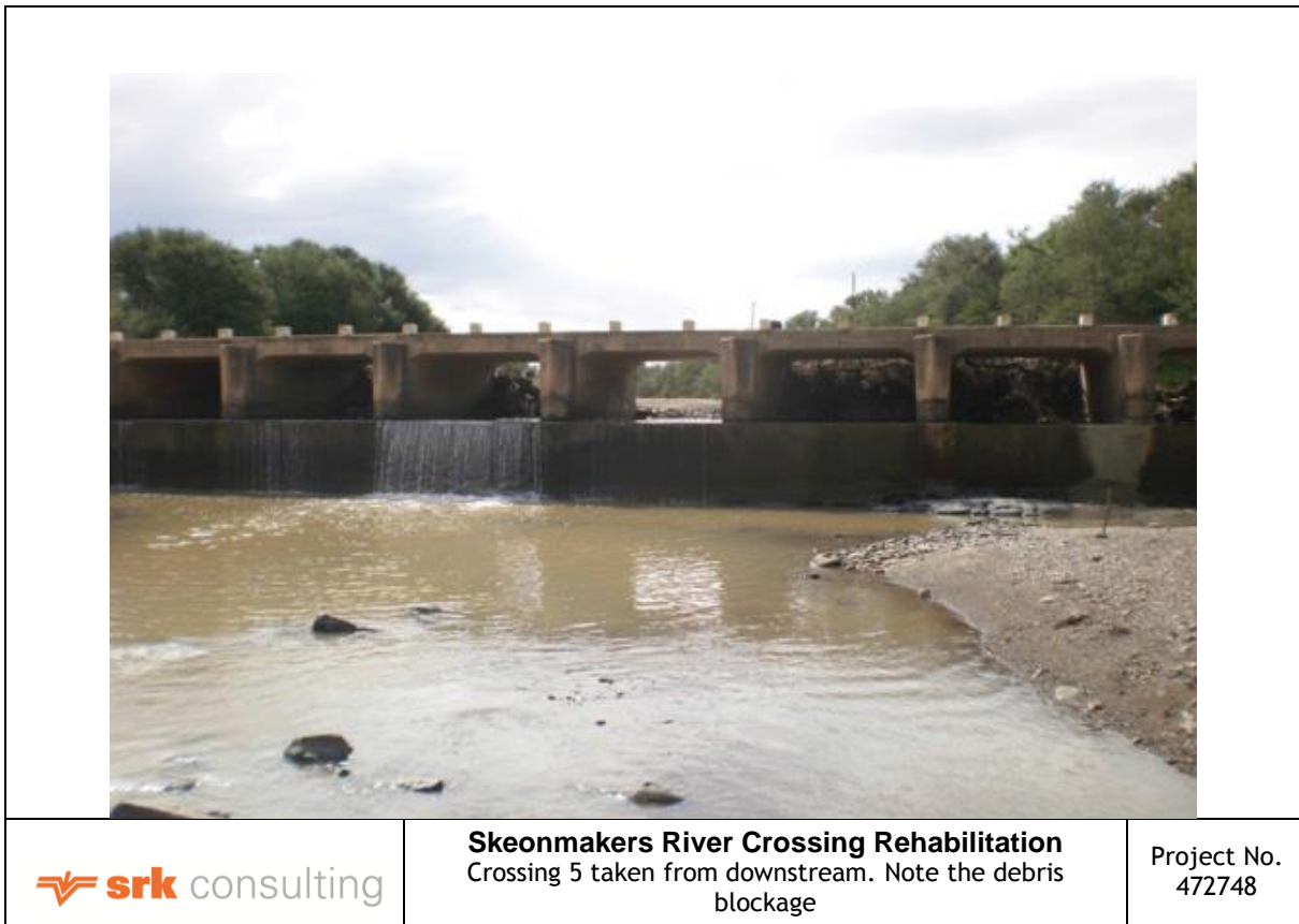
Figure 1: Crossing 5 taken from downstream. Note the debris blockage.
