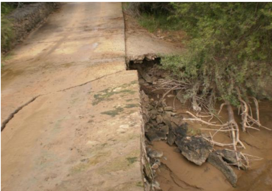
Figure 1: Crossing 8 taken from downstream. Note the damage on the left hand side.
