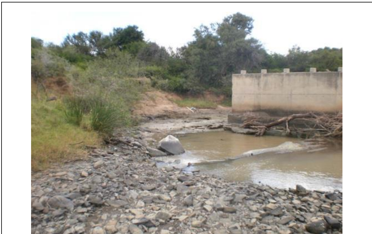
Figure 1: Crossing 4 taken from downstream. End cut washed away.
