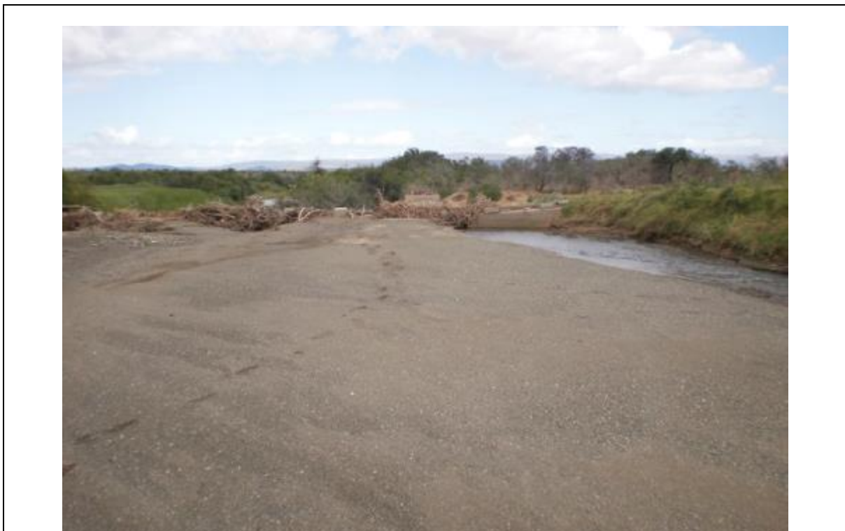
Figure 3: Upstream view. Note silt to top of slab
