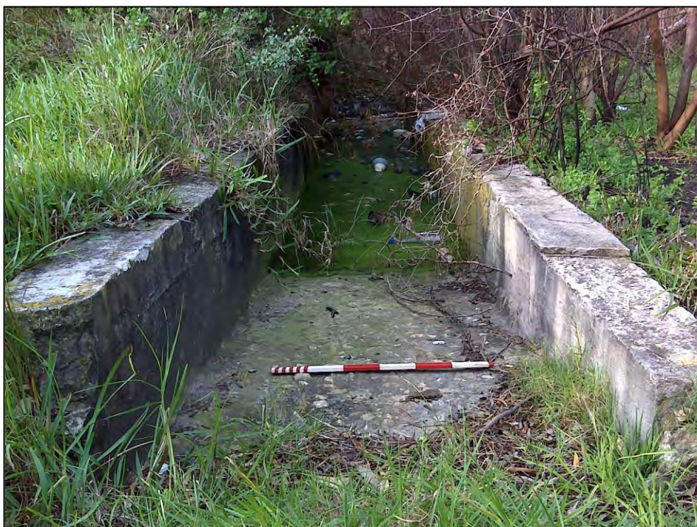
Figure 13. An unused dipping tank situated at QBE1.
