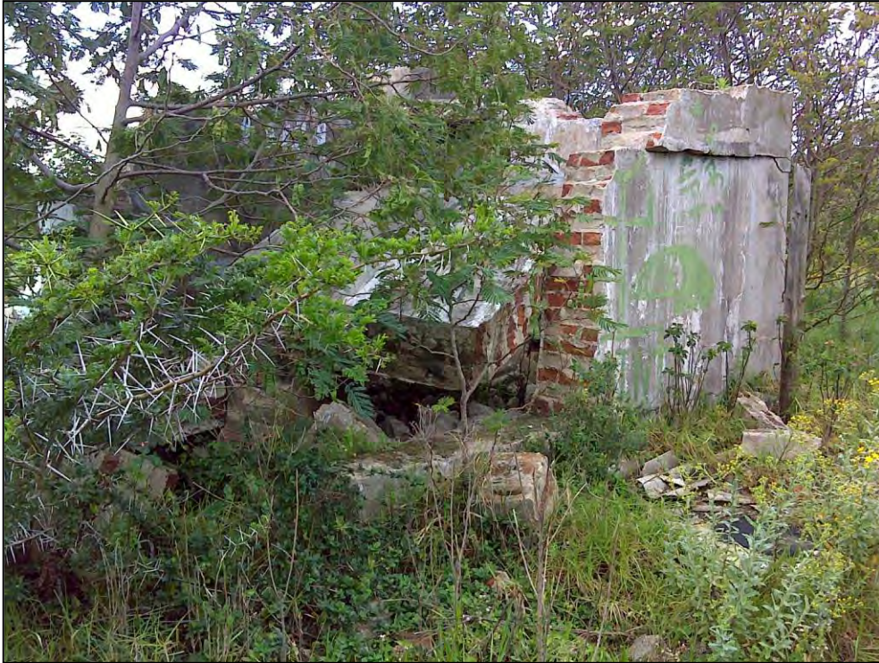
Figure 14. View of the ruin of a building situated at QBE2.
