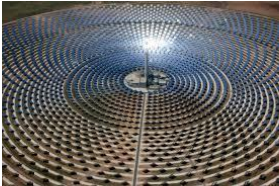
Figure 5-11: Elliptical formation of the Central Tower Solar Field (Source: www.finetubes.co.uk )
