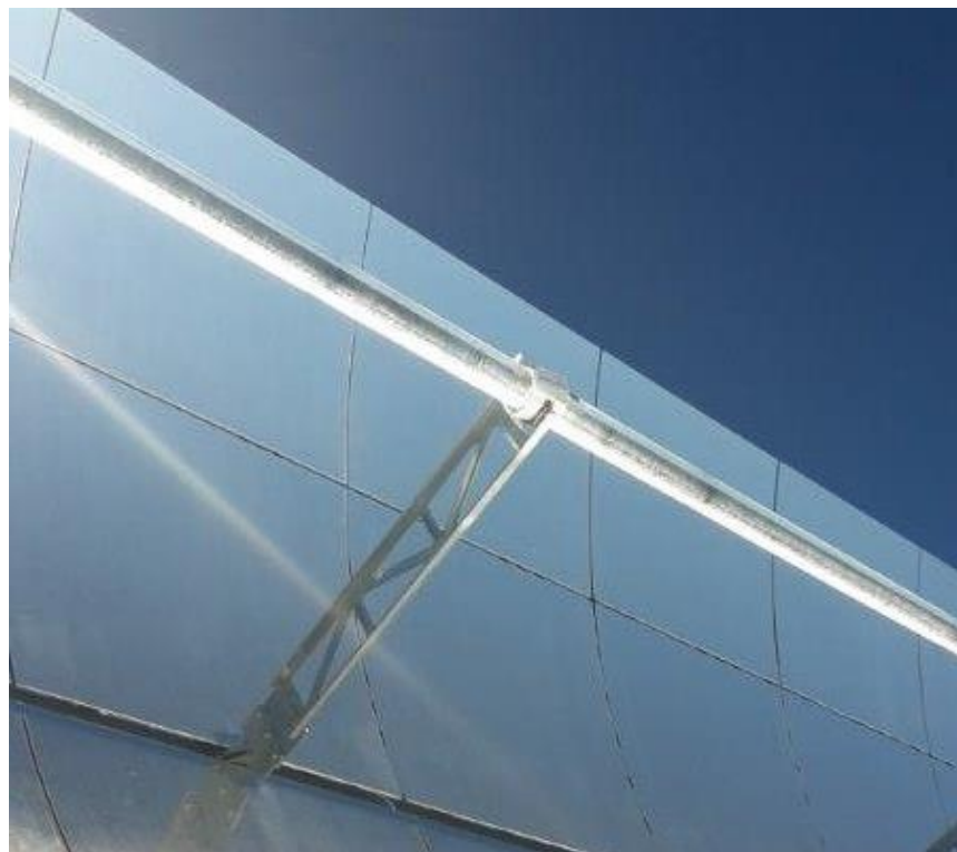
Figure 5-7: Parabolic Trough Absorber Tube (Source: WSP | Parsons Brinckerhoff)
