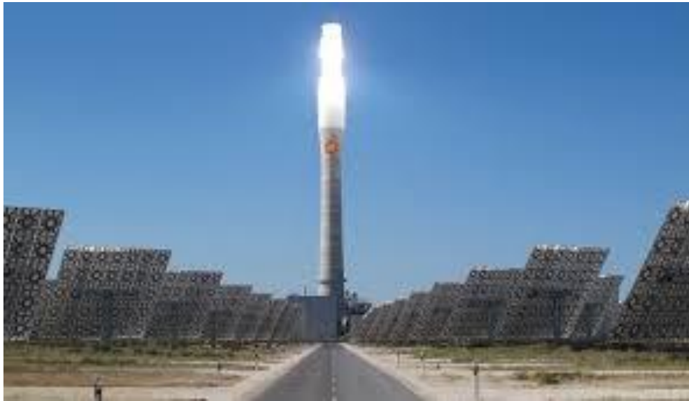
Figure 5-10: Central Receiver (Source: www.torresolarenergy.com )
