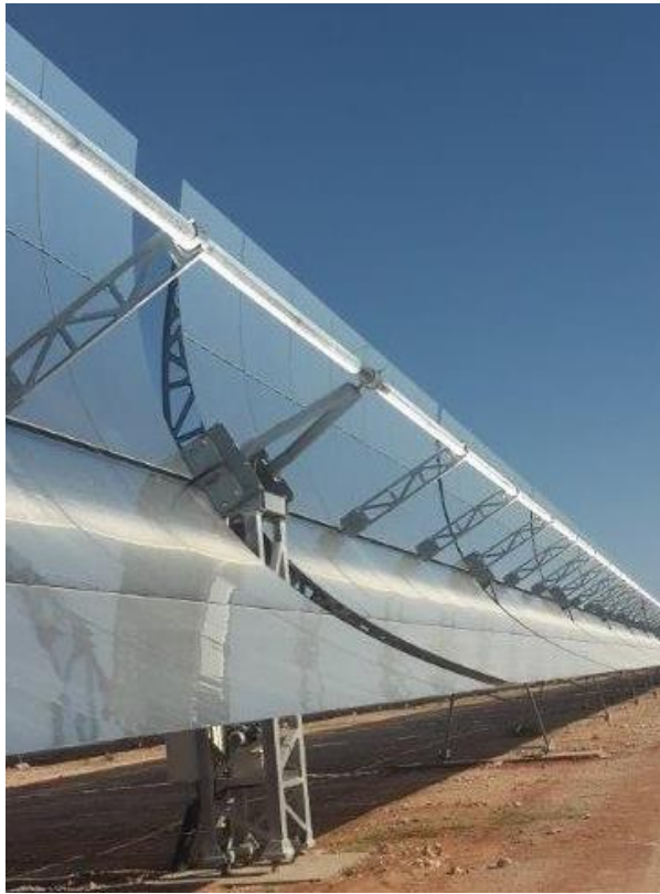
Figure 5-6: Parabolic Trough (Source: WSP | Parsons Brinckerhoff)
