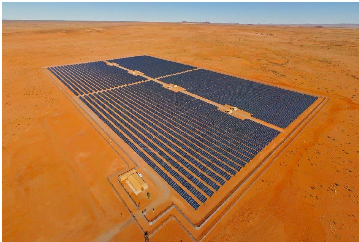
Figure 5-3: Large-Scale Photovoltaic Power Generation Facility
