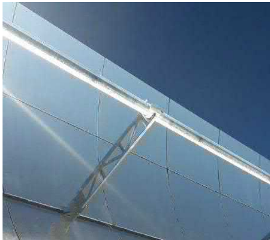
Figure 7-5: Parabolic Trough Absorber Tube (Source: WSP | Parsons Brinckerhoff)
