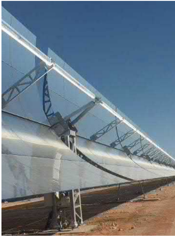
Figure 7-4: Parabolic Trough (Source: WSP | Parsons Brinckerhoff)
