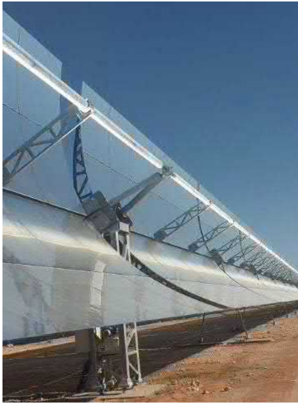
Figure 7-4: Parabolic Trough (Source: WSP | Parsons Brinckerhoff)
