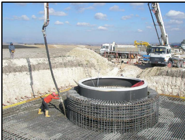
Figure 2-5: Concrete pouring of a turbine foundation – note the tower base collar in the foreground
