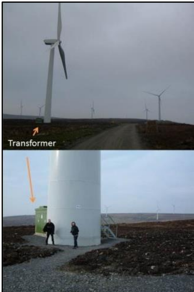
Figure 2-3: Photographs illustrating the external turbine step-up transformer
