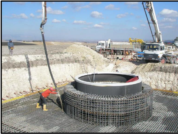
Figure 2-4: Concrete pouring of a turbine foundation – note the tower base collar in the foreground (CES, 2014)
