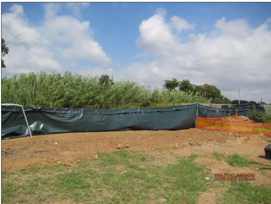
Figure 9 – Screening put up at the site to limit visibility from the outside as the area has a lot of foot traffic.
