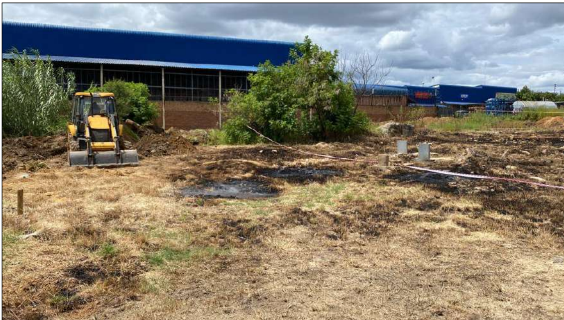
Figure 6 - General site view of the Hammanskraal graveyard. A TLB is busy digging trenches to divert the water.
