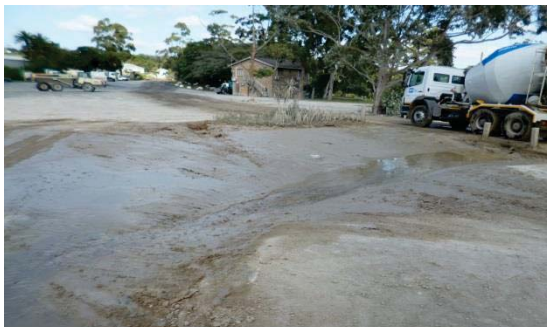
Plate 23: Concrete plant drainage channel, reporting to the treatment facility.
