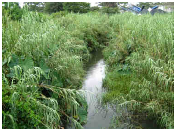
Photo 15. View of the partially blocked channel with dense aquatic vegetation growth just upstream of the road bridge in Photo 17.
