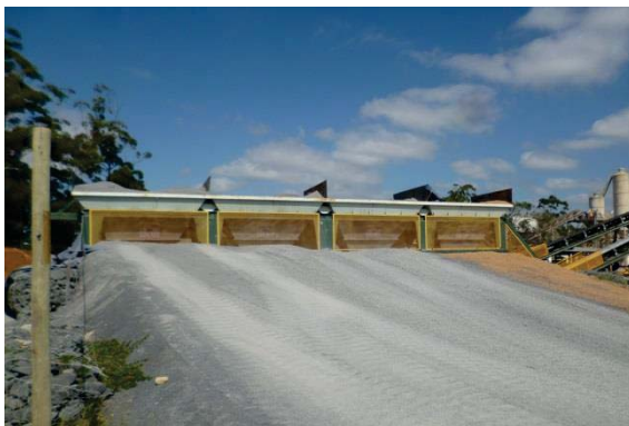
Plate 9: Ramp Up to Cold feed bins of the Asphalt Plant.
