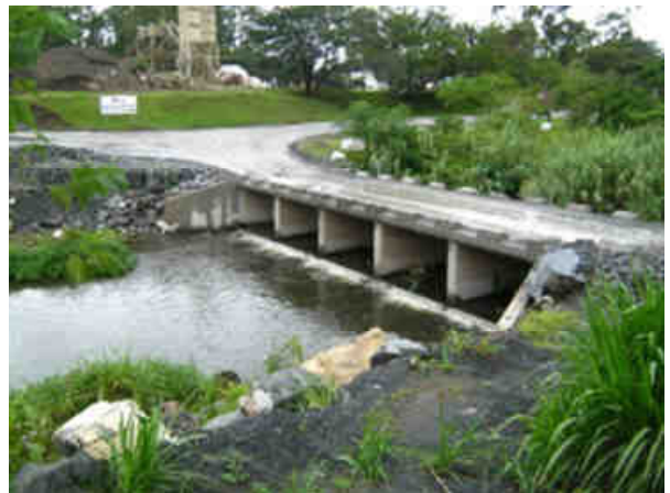
Photo 17. View of bare unstable river banks below the lower road bridge crossing. Gabions used to stabilise banks are broken or incorrectly packed, keyed-in and tied.
