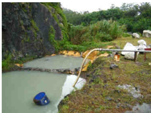
Photo 18. View of the existing storm water detention/settling ponds used to store contaminated runoff. The water is normally pumped from the ponds and used for dust suppression at the quarry and is not permitted to discharge into the adjacent Vungu River unless via overflow during storm events.
