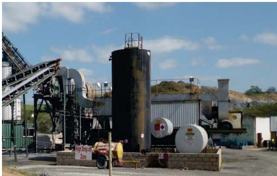
Plate 11: Bunded Asphalt and Diesel AST tanks.
