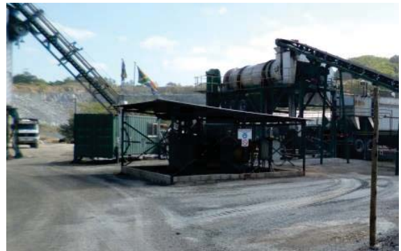
Plate 12: Generator for asphalt plant, under roof cover and bunded.
