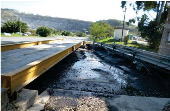
Plate 3: Runoff from weigh bridge and offices reporting to existing channel, at the Weigh bridge area.
