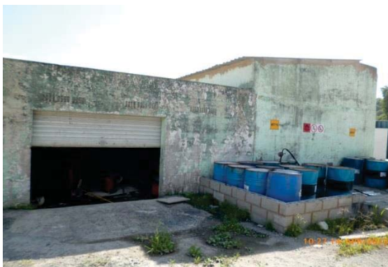
Plate 15: General Storage area under roof cover, with bundled storage area for Wet Fix and Econat.
