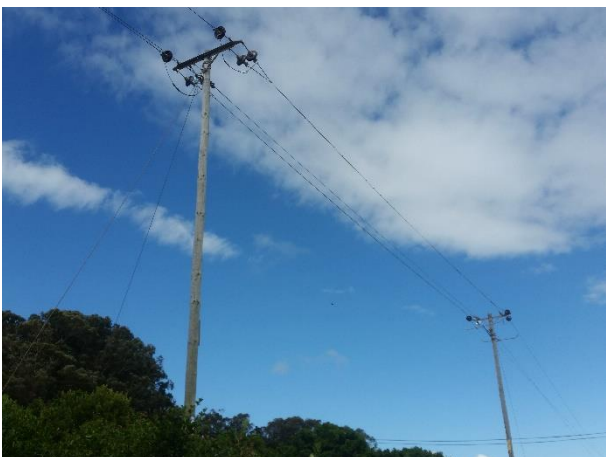
13: Close-up of the powerline crossing in photo 12
