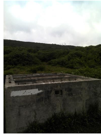
GM1-1: Broken infrastructure on the existing Churchill pipeline alignment Photo 40
