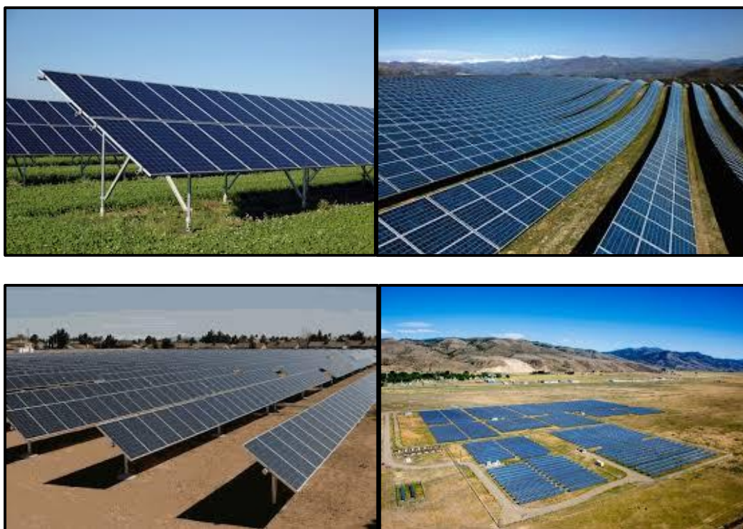
Figure 2-9: Examples of what typical PV arrays might look like
