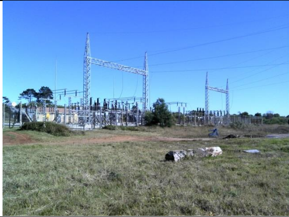
Photo 1: Existing Lorraine 132 kV Substation
