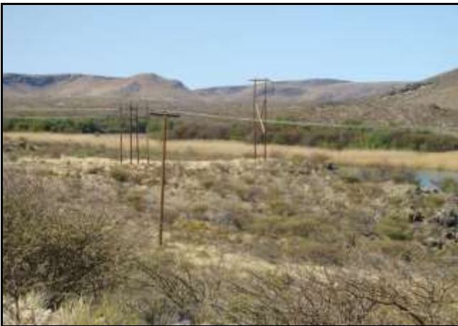
Figure 7: The point where the power line would cross the river alongside an existing line.
