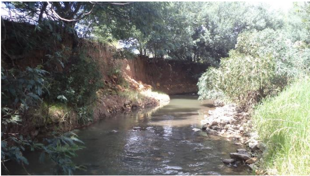
Figure 10: Upstream view of the CK2 site indicating the severe bank erosion and invasion by Acacia mearnsi at this point (February 2014)
