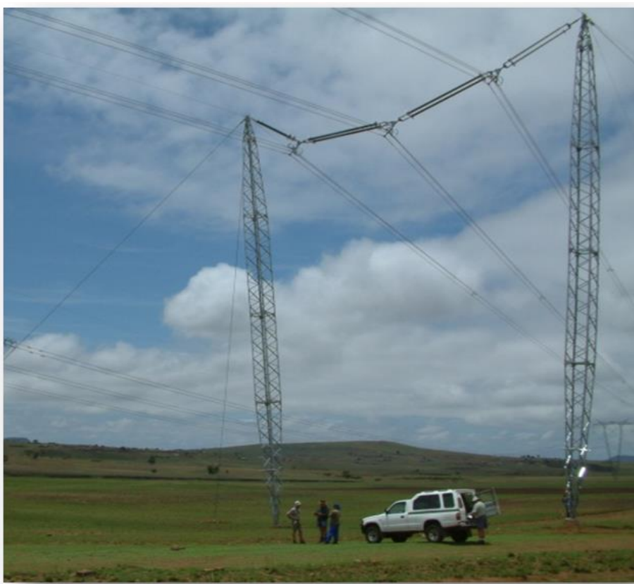
Plate 1: Cross Rope Tower
