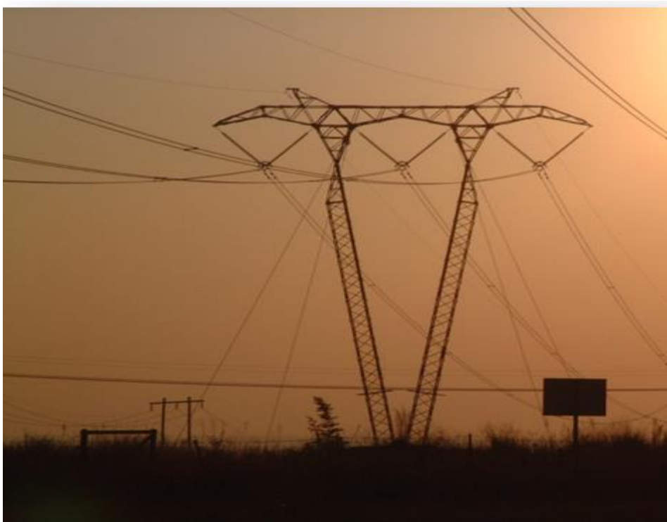
Plate 3: GUYED VEE Tower
