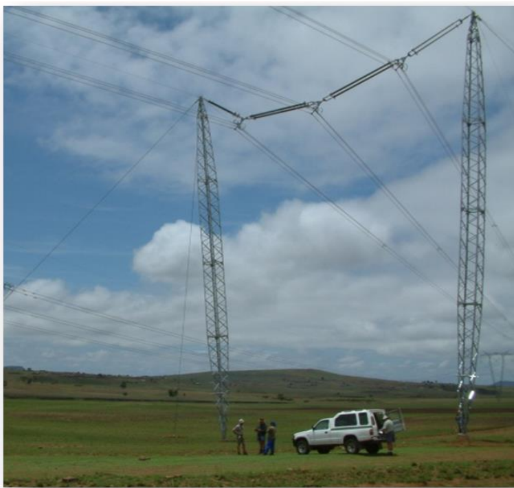
Plate 1: Cross Rope Tower
