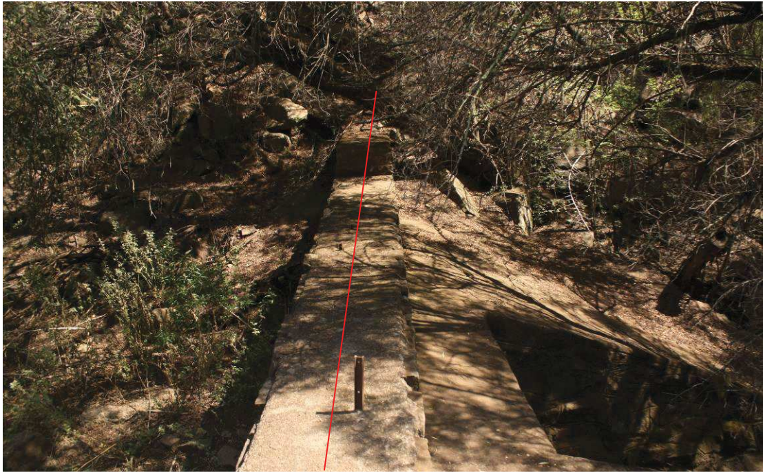
Figure 3: The weir within the stream on which the pipeline will be attached (red line).
