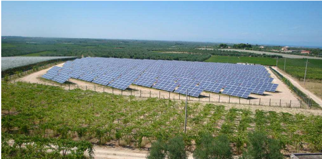
Figure 3: Installed PV Panels (Sourced from Ecoware)
