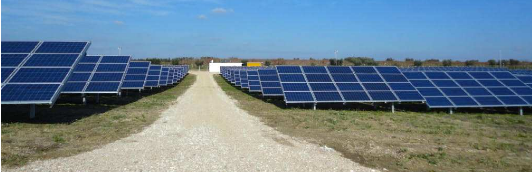
Figure 2: Installed PV Panels (Sourced from Ecoware)
