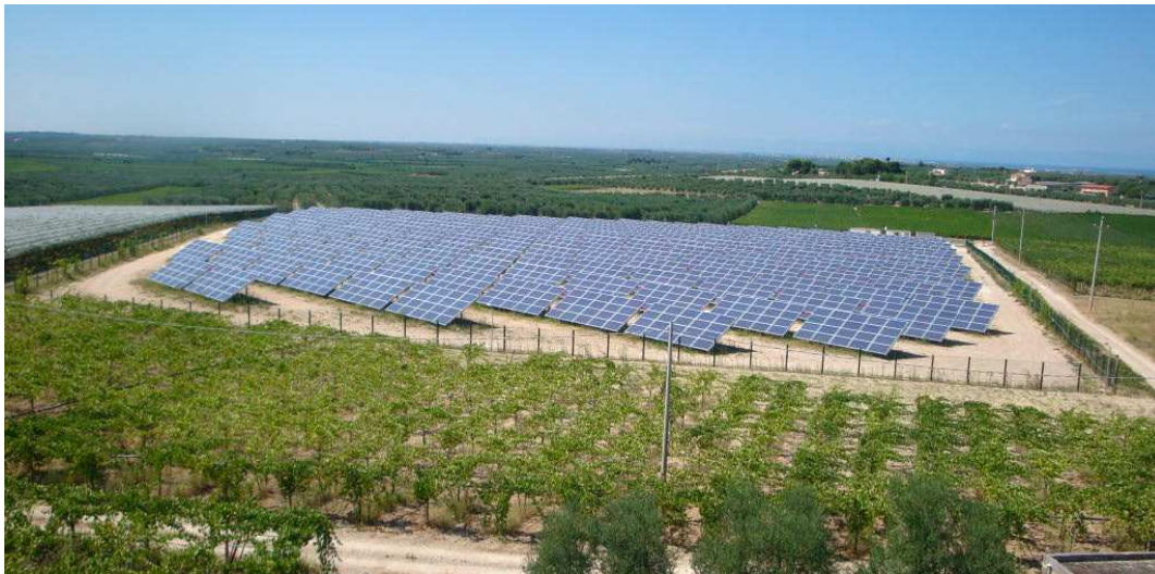
Figure 3: Installed PV Panels (Sourced from Ecoware)
