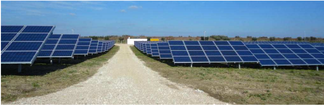
Figure 2: Installed PV Panels (Sourced from Ecoware)
