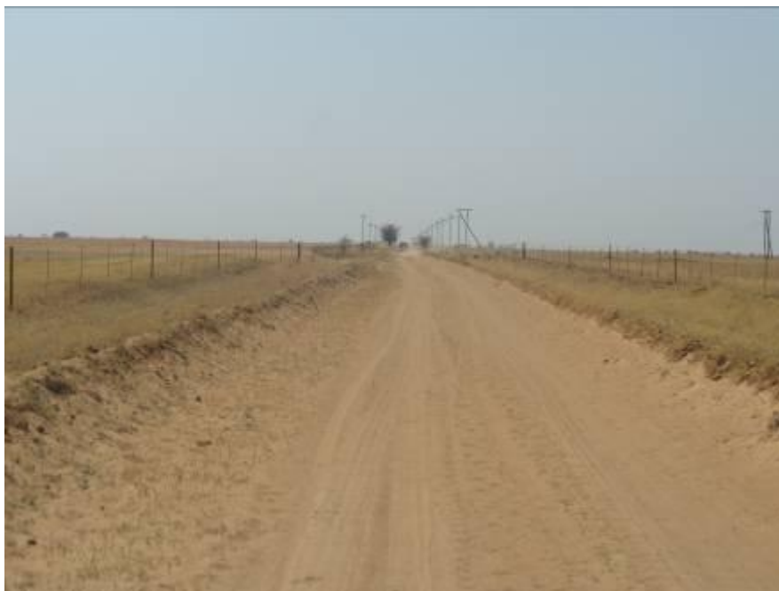
Figure 7, Dilapidated unclassified farm road.
