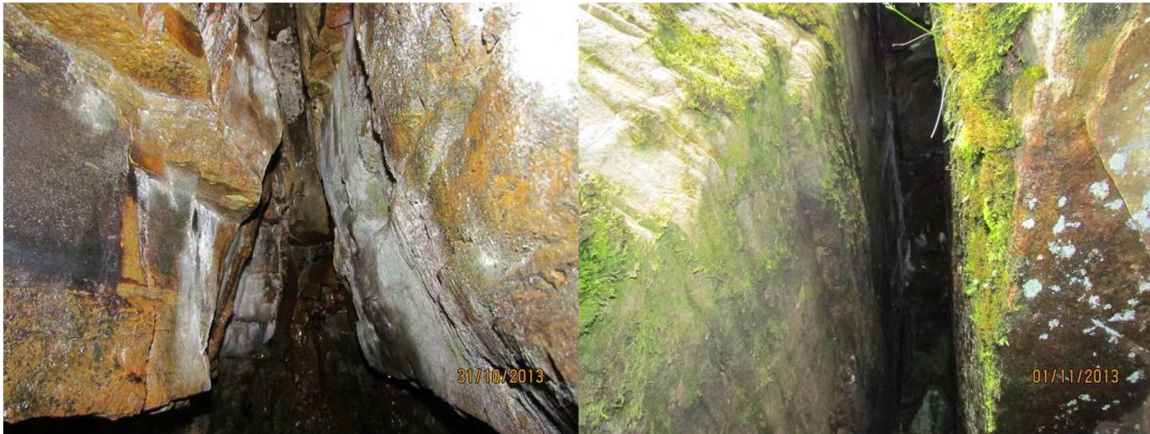
Photograph 10: Numerous caves and crevices which are likely to provide roosting sites for various chiroptera species were recorded on the cliffs associated with the proposed development
