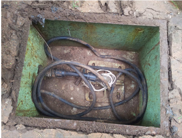
Plate2: BH03: Equipment on the outlet (submersible pump)
