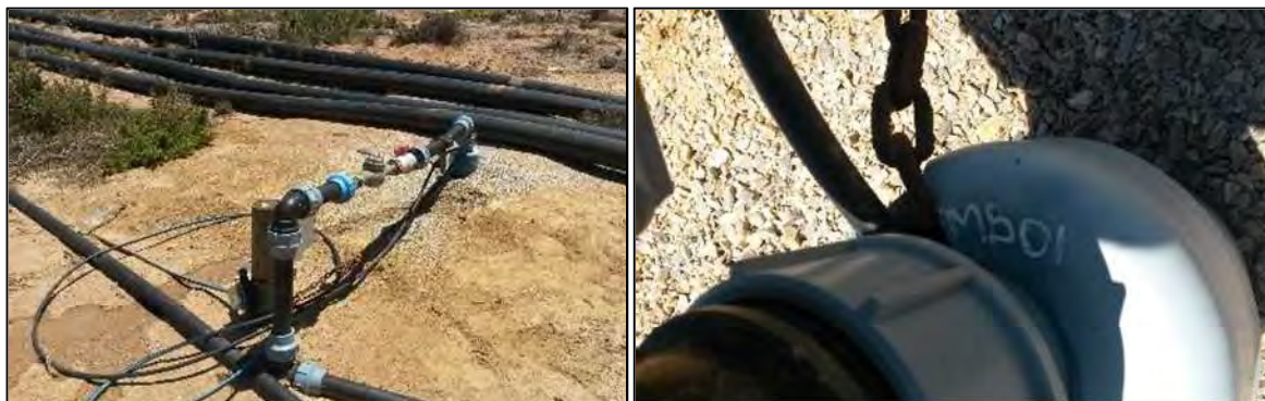
Figure 33: Borehole TMB01 – unable to measure water level and no longer in use
