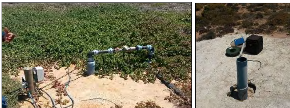
Figure 34: Borehole TMB04 – unable to measure water level and no longer in use (left) and Borehole TPB01 – dry to 30 m (right)
