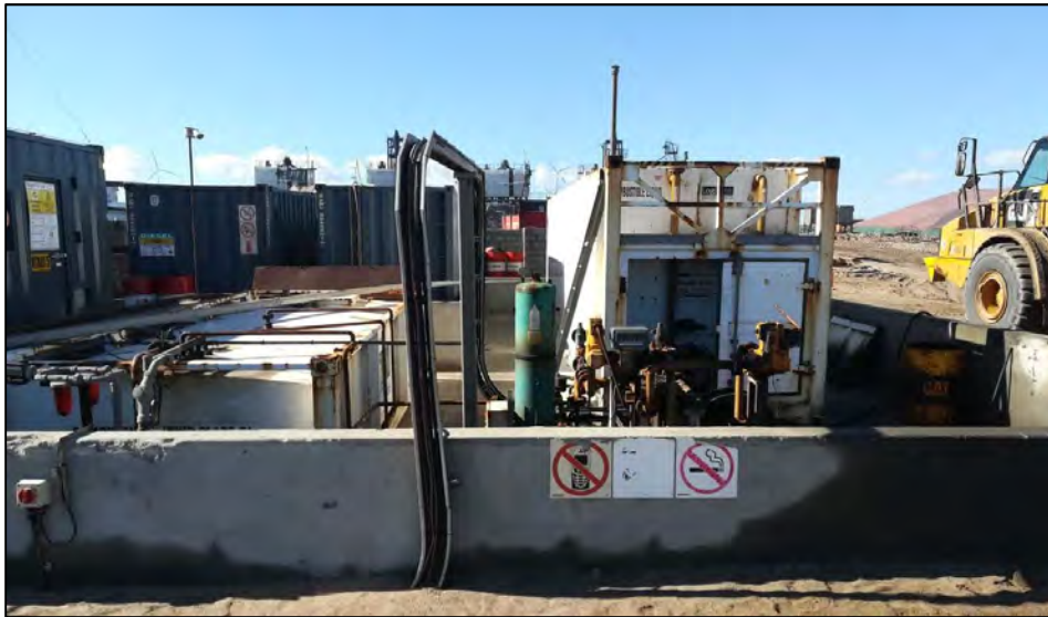
Figure 20: Diesel storage area
