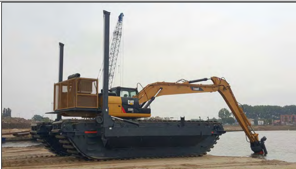
Figure 11: Example of an excavator and slurry pump potentially to be used by MSR on the beaches
