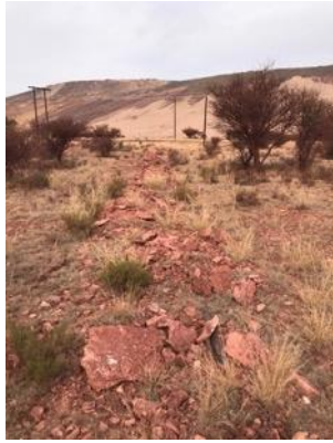
Figure 19: Sunken pipeline in the area adjacent to the proposed railway line.
