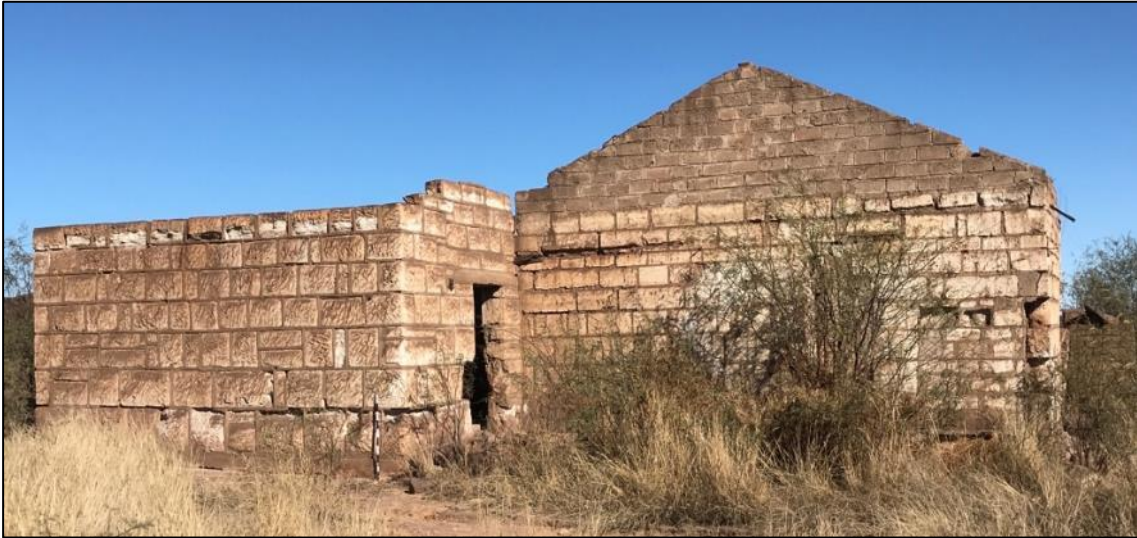
Figure 66 – Another view of the structure at site YORK-001. Note the cut stone walling with gable likely constructed of cement bricks.
