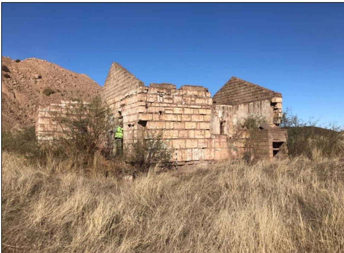
Figure 65 – General view of the structure at site YORK-001. Note the walls of neatly cut stone masonry with gables likely constructed of cement bricks.
