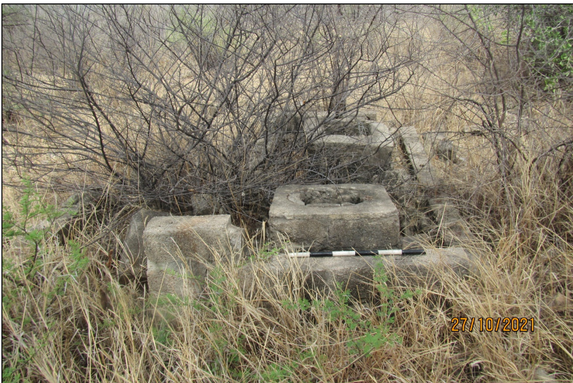
Figure 26 - View of the remains of a toilet.
