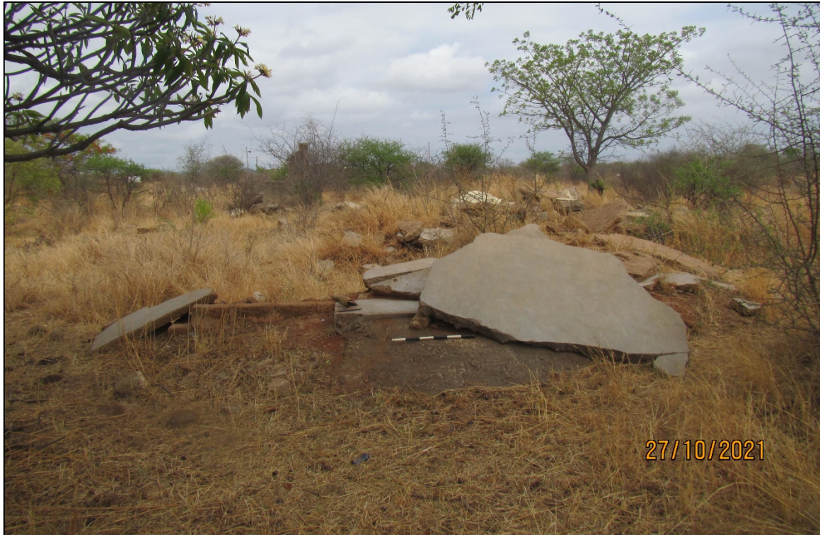
Figure 23 - View of the collapsed walls of one of the structures. The scale is in 10cm increments.
