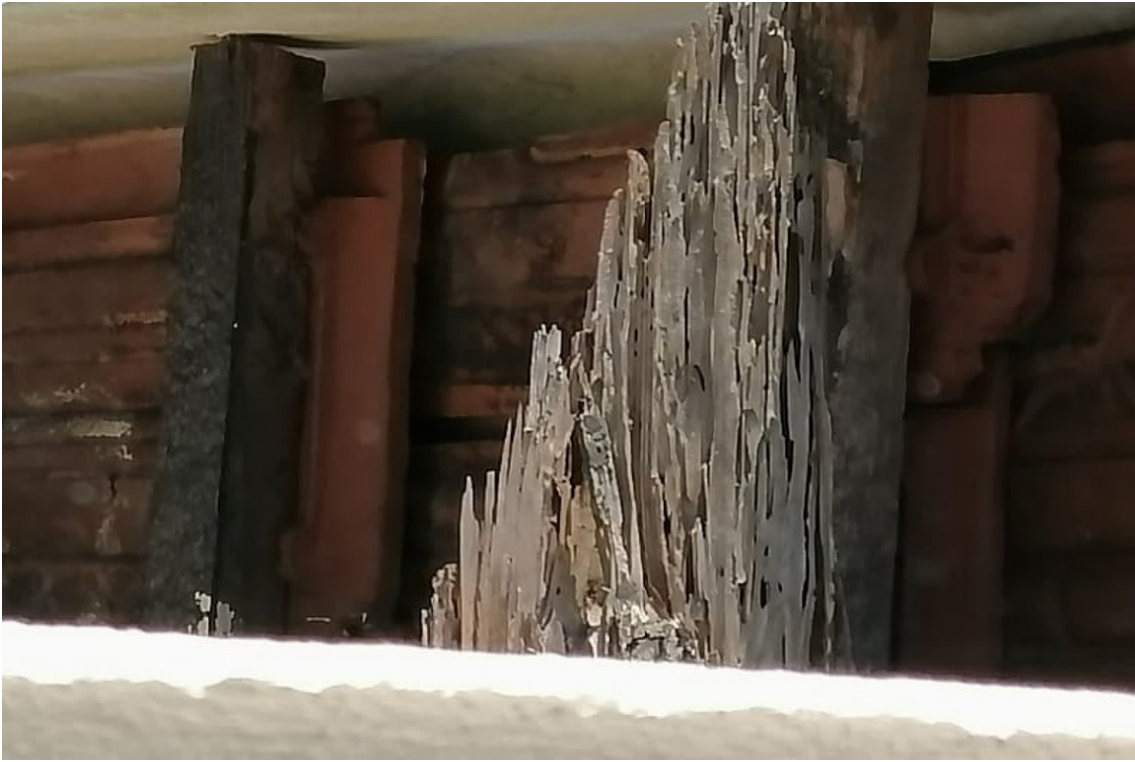
Structurally damaged timber roof trusses.
