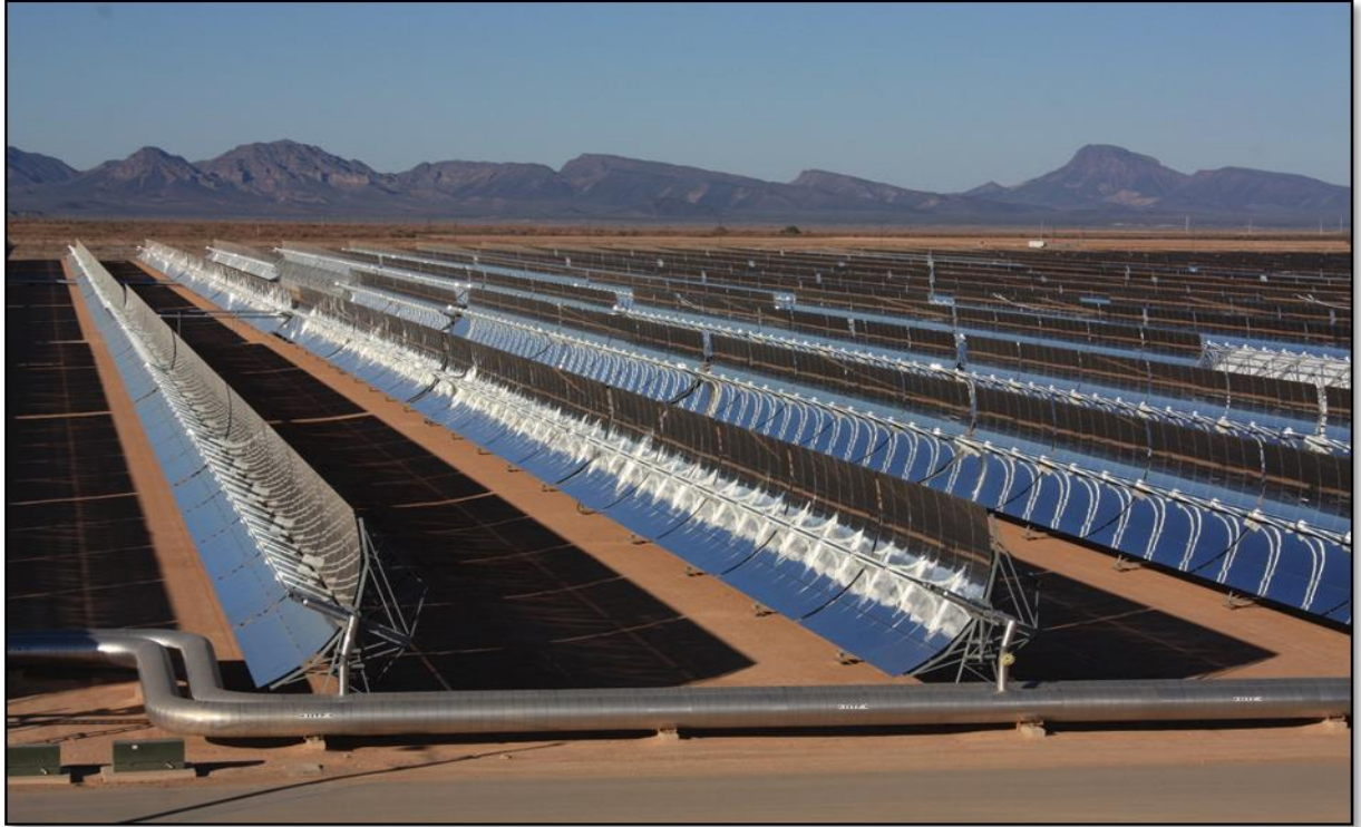
Figure 1: A typical example of a Parabolic Trough System.
