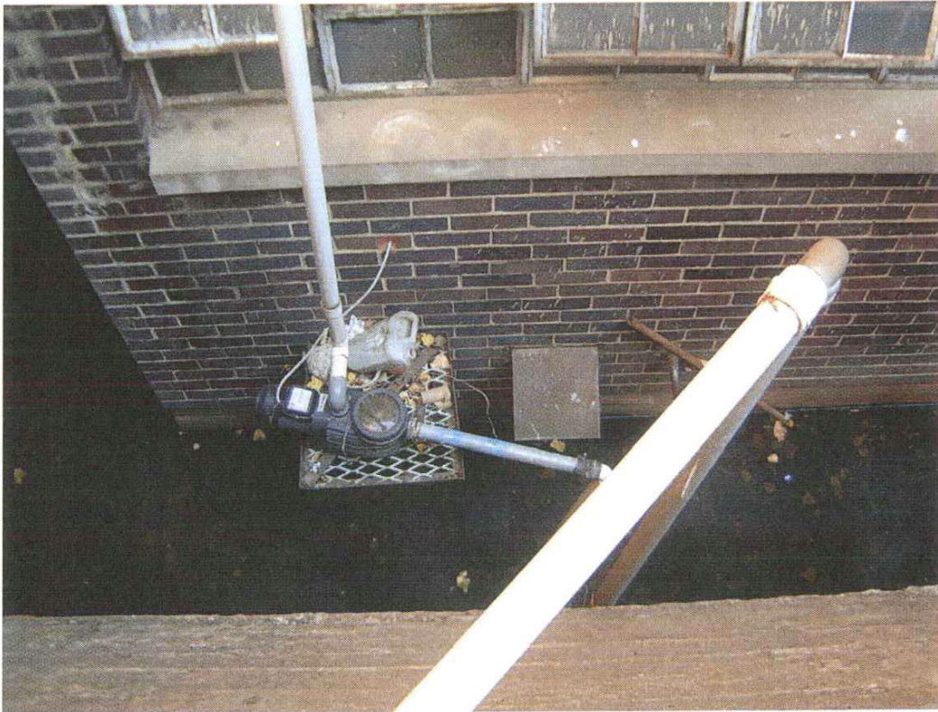
Photograph 5: Water at basement level. Pump used to deliver water to ground level.
