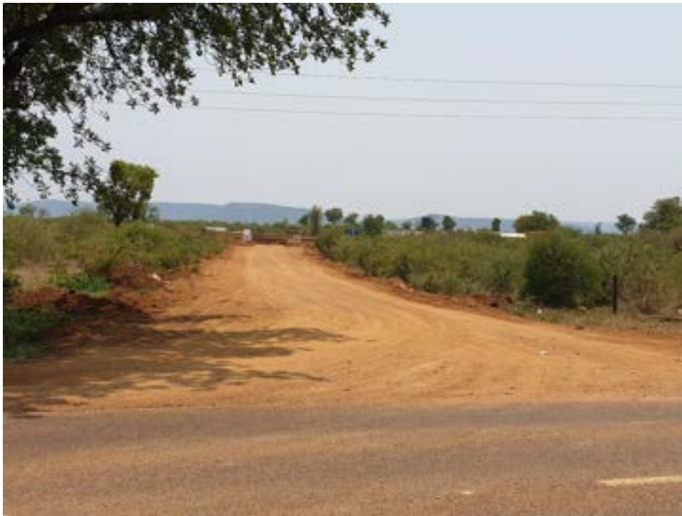
Photo 5: Deviation 3 facing West, the construction vehicles are busy constructing the Pennigotcha and Mhingaville substation located along Punda Maria road R524.
